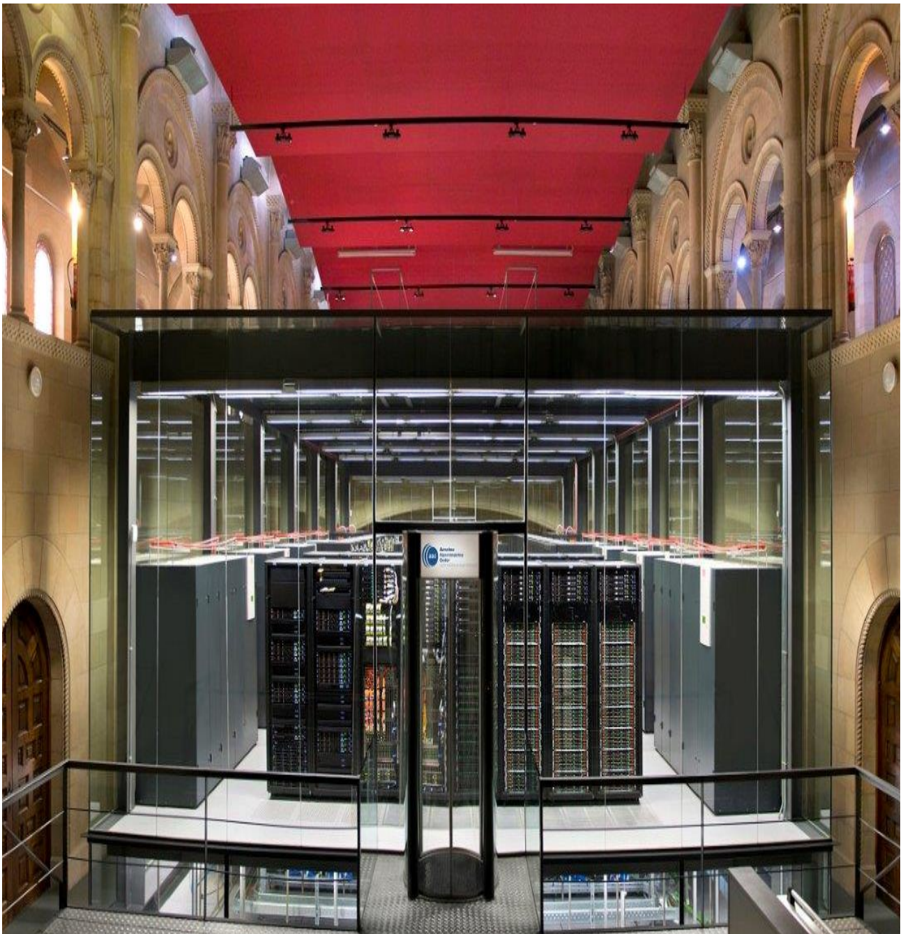
Barcelona Supercomputing Center
